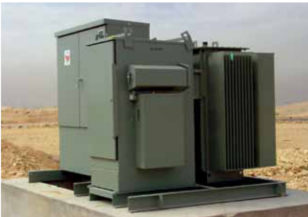
Scimitar SFRMU Transformer Mounted
