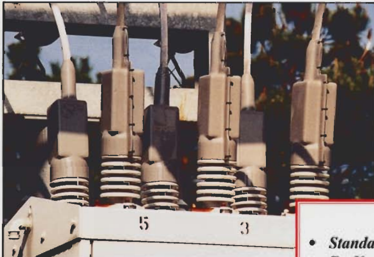
Reusable Insulating Boots encapsulating cable joints and terminations on 27kV outdoor circuit breaker.
