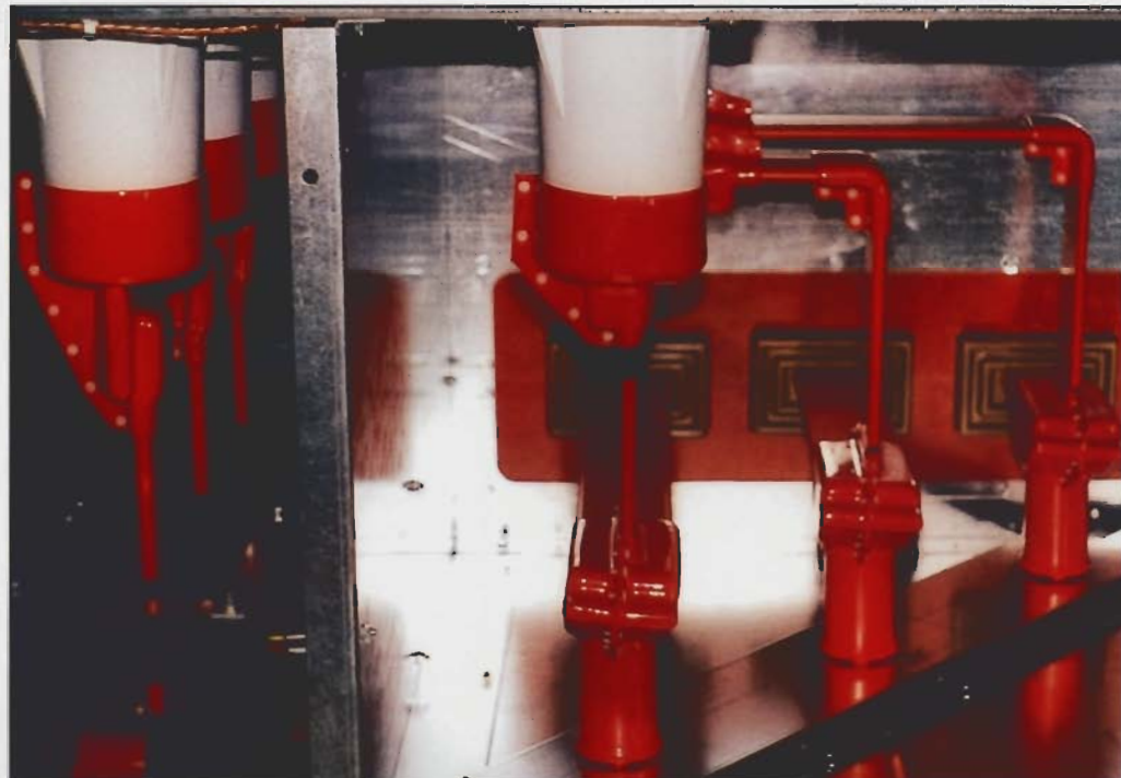
Form Fitting Insulating Boots in 15kv medium voltage metalclad switchgear.
