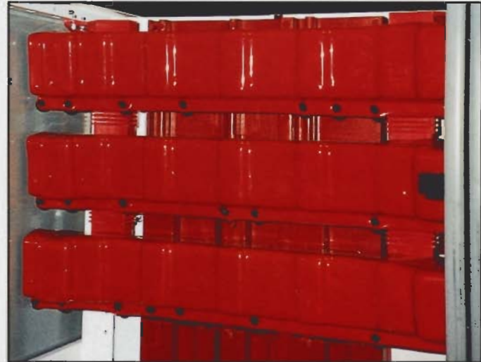
Insulating Boots encapsulating the busbars of a 600 volt low voltage Multi-Motor Control Board.
