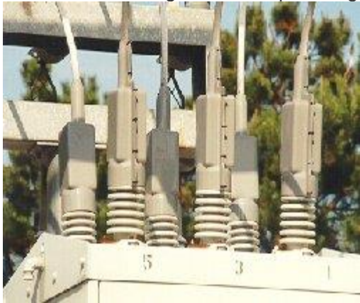
Reusable insulating boots encapsulating conductor terminations on outdoor circuit breaker.
