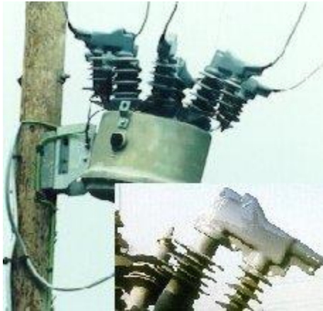
Insulating boots encapsulating cable joints and terminations on a pole mounted medium voltage recloser unit.
